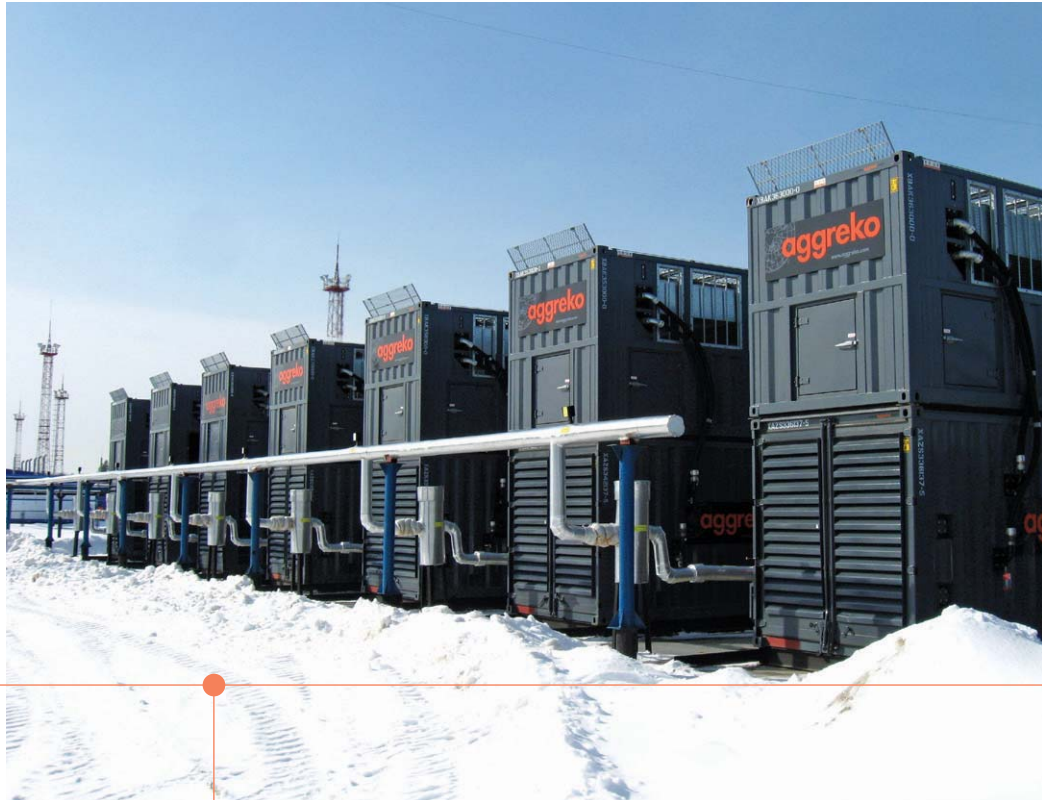
Gas installation at Taylakovskoye oil field in Western Siberia
